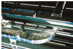
1286 1287 Figure 6.2.13. Cable tray wrapped in fire barrier mat. 1288 Photo courtesy of 3M. 1289
