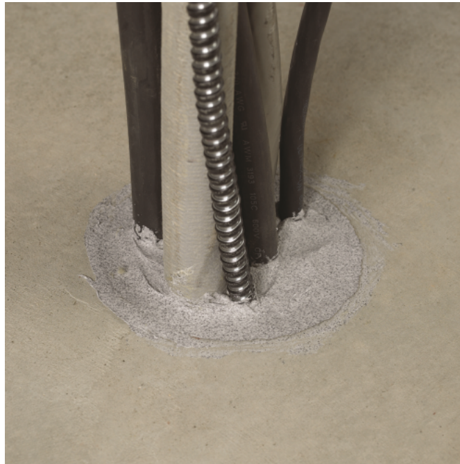
898 899 Figure 6.2.1.2. Firestop sealant applied to floor penetration. 900 Photo courtesy of 3M.
