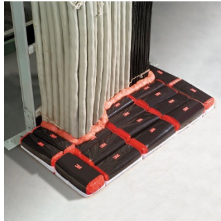
754 755 Figure 5.6. Large opening closed with fire barrier pillows and putty. 756 Photo courtesy of 3M.
