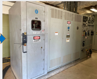
To 480V Low Voltage Switchgear
