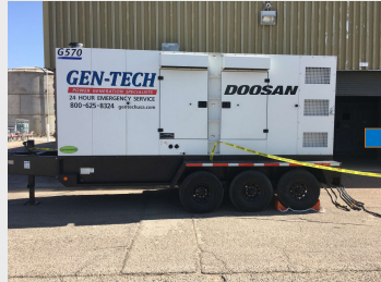
Connect 480V, = 500 kW, 3-Phase Generator
