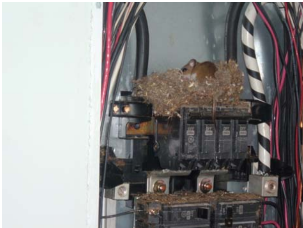
Mouse In A Panelboard
