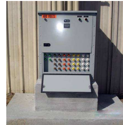
3200 Amp @ 480 Volt (2000kW) Generator Connection Cabinet - Access Door open showing Cam Lock connections
